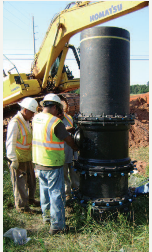
Construction on the Tussahaw Transmission Main, which runs east to west through Henry County and connects the Authority's two water treatment plants, was recently completed to provide system flexibility and redundancy in water distribution, allowing for easier plant maintenance without service interruption.
